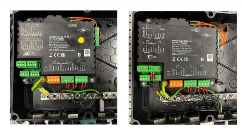
CM-RC-02 in protection mode (left) and compressor operating mode (right)
